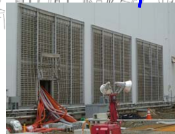
3u Emergency D/G air inlet louver
